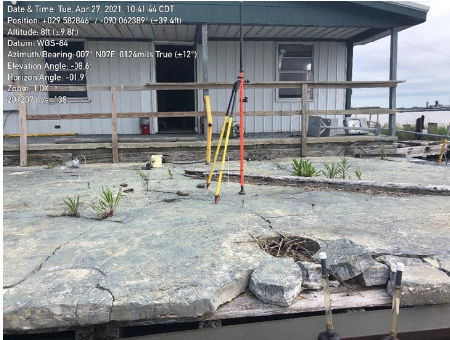
Figure 6. Checkpoint NVA_138. This checkpoint is located on a concrete dock. Review by Dewberry deemed this survey checkpoint unsuitable to use in the swath vertical accuracy testing.
