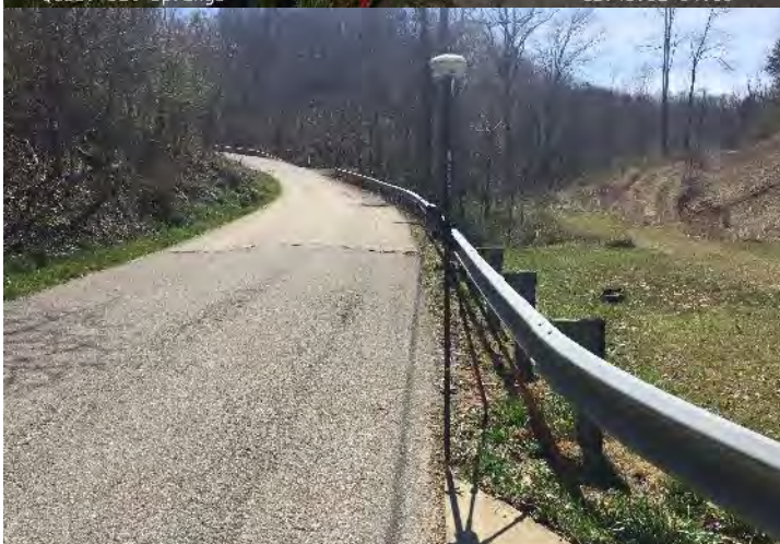
JD091 R033656 KY_Cal052 Pavement 2019-04-01 12:48:24-04:00 Quad: Oil Springs
