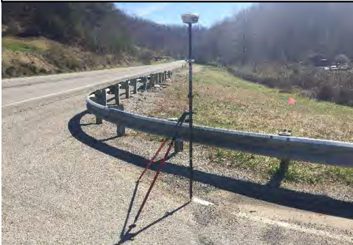
JD091 R033656 KY_Cal055 Pavement 2019-04-01 11:21:55-04:00 Quad: Oil Springs
